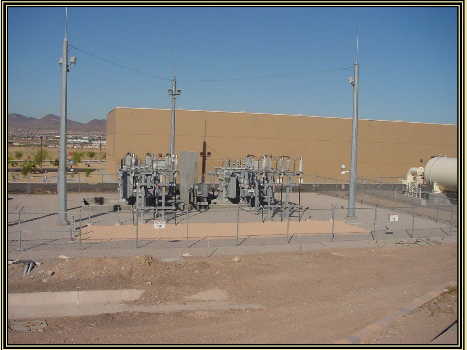
RMPS-B 69/4.16KV Distribution Substation
